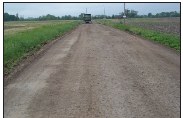
The road was opened to traffic immediately after the work was completed. The county will come back in the next few weeks to seal the road using the chip and seal process.
