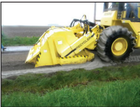
BOMAG™ reclaimer, courtesy of Southeastern Equipment, preparing the road prior to rolling out the grout mix
